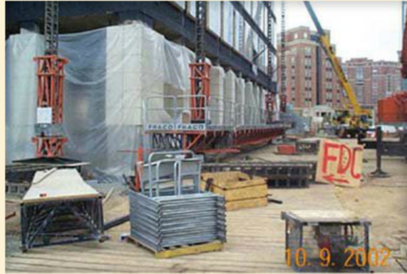
Figure 8-2 Fire departments have a vested interest in regulating construction, as evidenced by this blocked fire department connection at a construction site.
