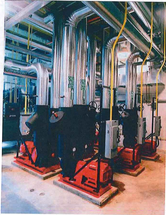
FIGURE 8.16 Photograph of Mechanical Piping
