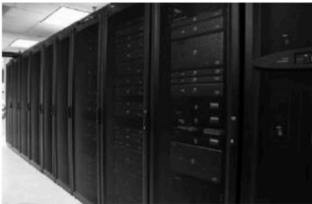
FIGURE 8-4 The blade server is designed to fit within a rack with other blade servers. This reduces the server's physical footprint, makes the server easier to cool, and reduces the server's power consumption.
