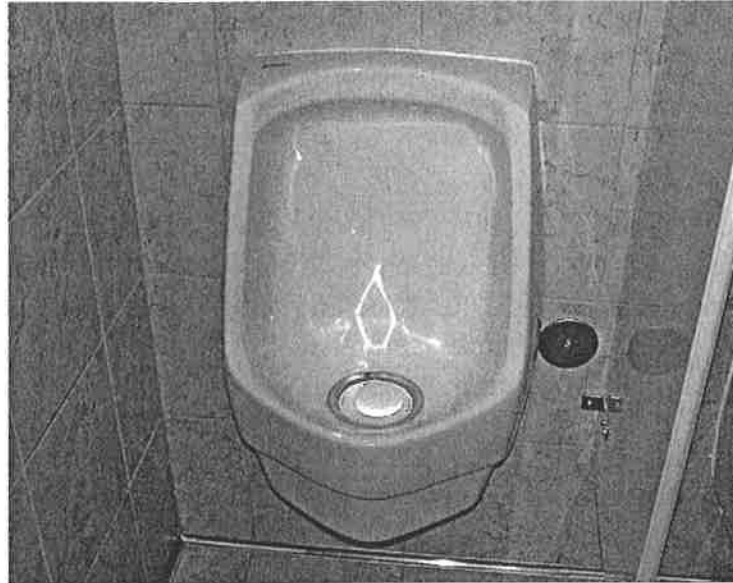
Figure 2-1: Waterless urinal. This is a waterless urinal at the EPA Region 8 Headquarters. While such urinals have benefits for the environment, they can present maintenance problems when not properly designed to make them easy to use and service.
