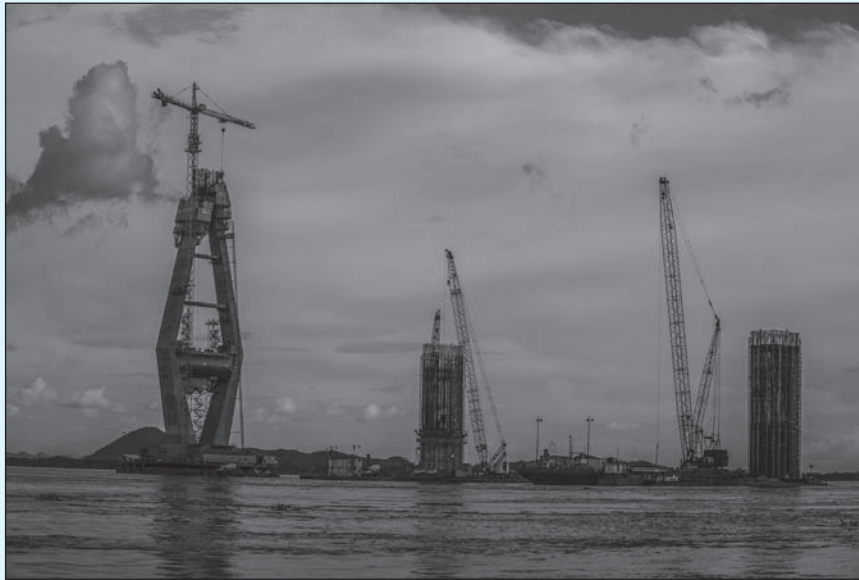
Unfinished Mercosur Bridge in Caicara del Orinoco, Venezuela, an Odebrecht Project
