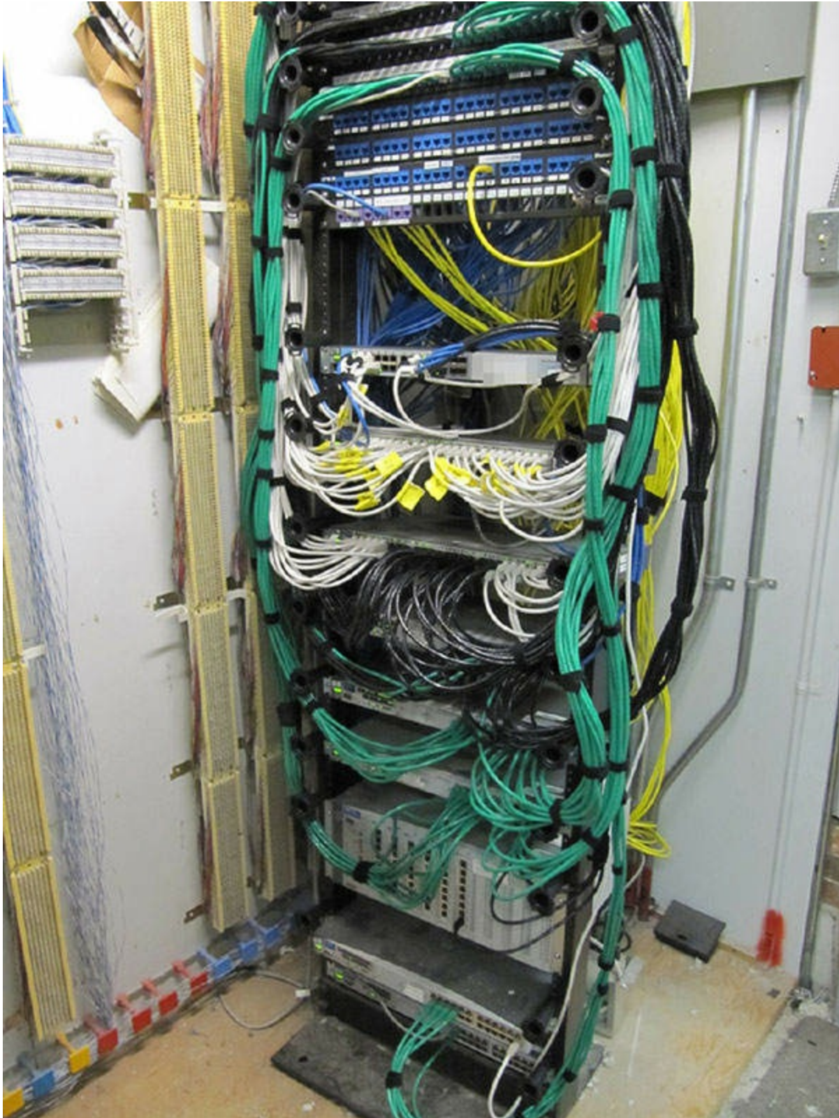
FIGURE 10.1 A typical wiring closet
