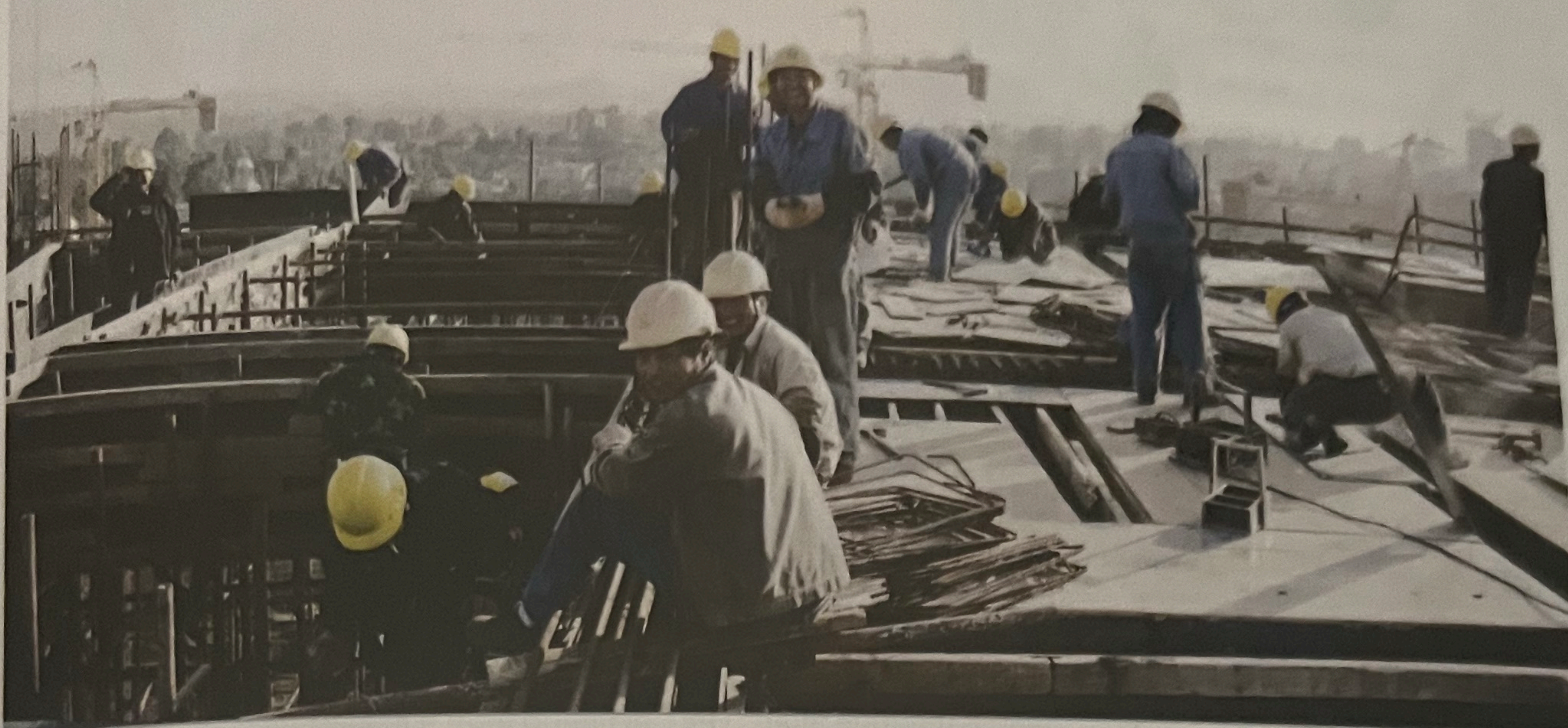
Chinese construction workers build the new African Union Buildings in Addis Ababa, Ethiopia.
