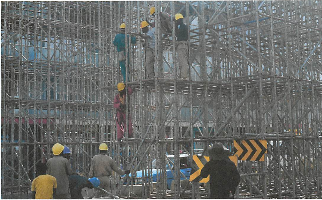
THE BUILDING OF INFRASTRUCTURE IN AFRICA, LIKE THIS LIGHT RAIL NETWORK BEING BUILT IN ADDIS ABABA BY A CHINESE COMPANY, IS ESSENTIAL FOR PROMOTING TRADE AND DEVELOPMENT.
