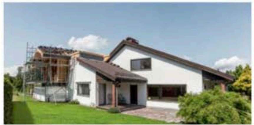
▲ Figure 36.1 If building work starts without planning permission, a council can issue a prohibitory injunction
