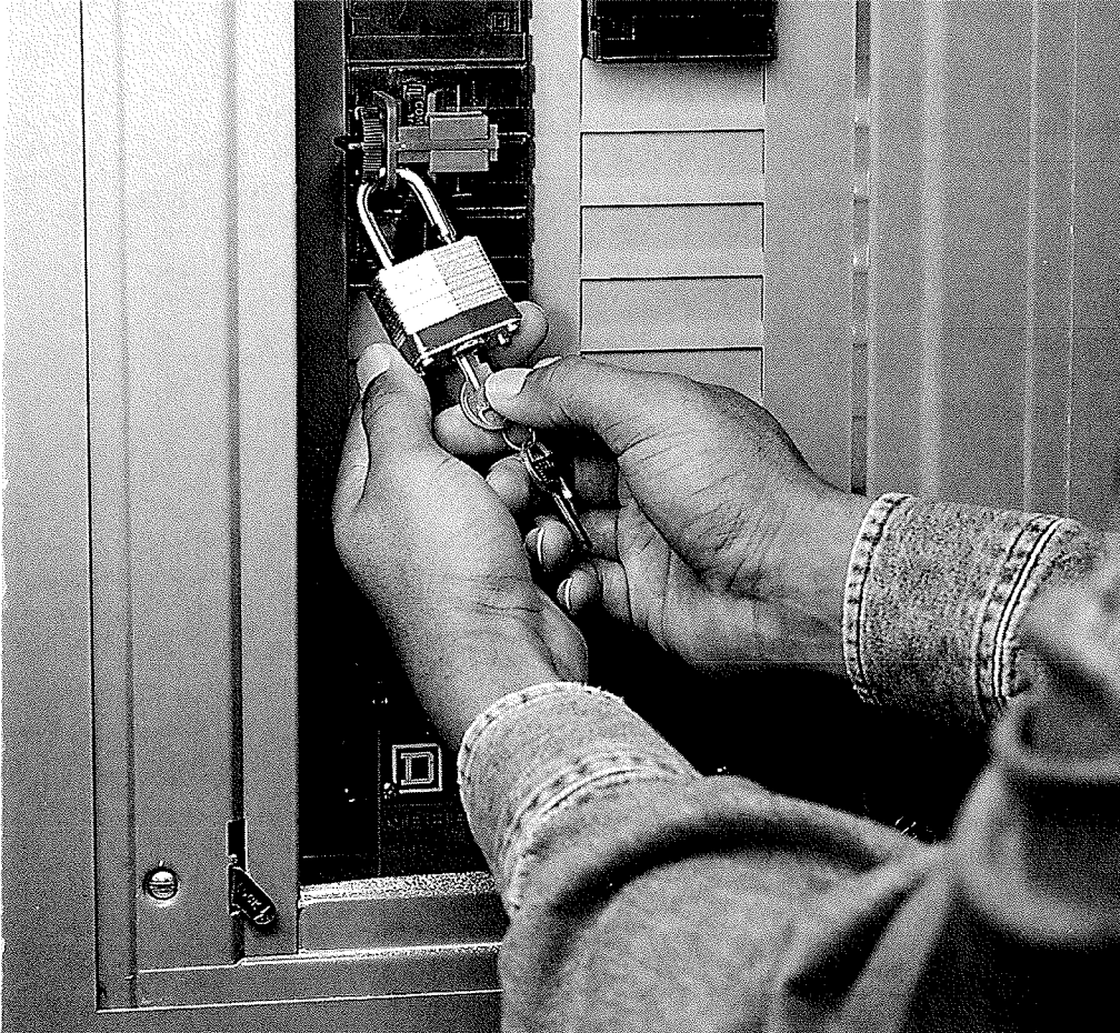
Lockout/tagout at a circuit breaker.
